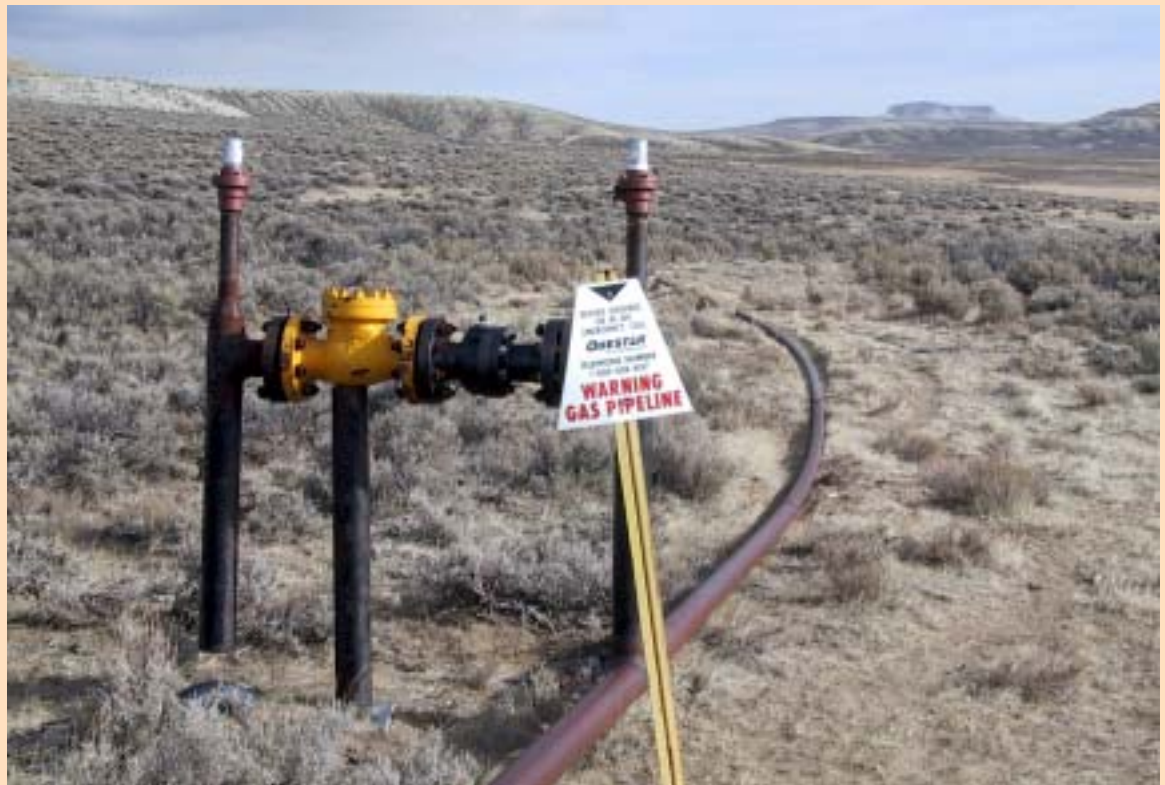
Gas Pipeline in the Uinta Basin
